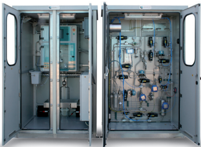
Analyzer shelter with integrated sample preconditioning system
