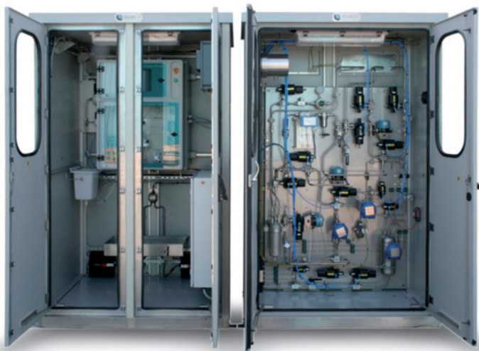
Analyzer shelter with integrated sample preconditioning system
